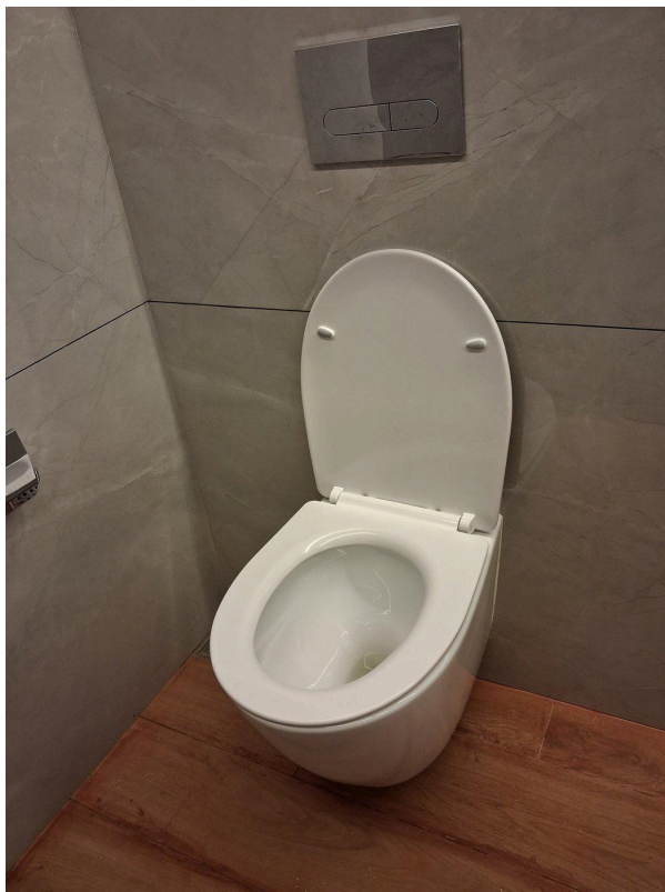
Accessible (Comboard) Toilet — Fixture
